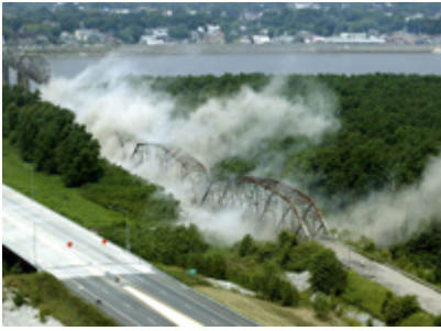
Razing of old highway bridge across the Mississippi River created a more powerful than expected back-blast for photographer and camera gear on the ground. Photo courtesy of Southeast Missourian.
